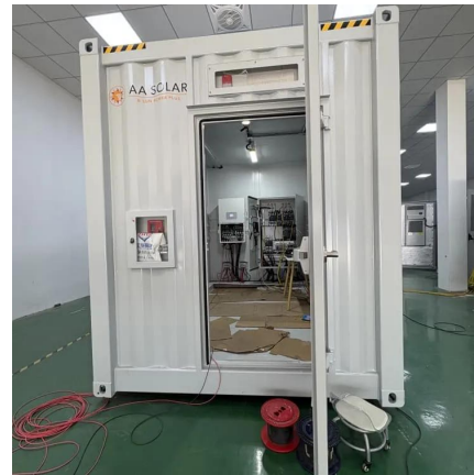
Energy storage container, BESS container
