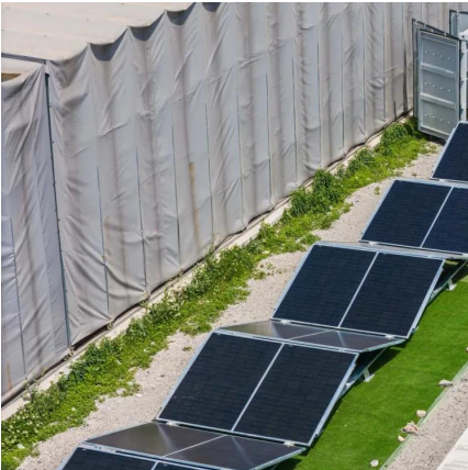
Solar + Battery Storage Installation Toronto
