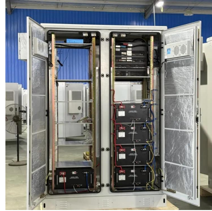
Energy storage container, BESS container
