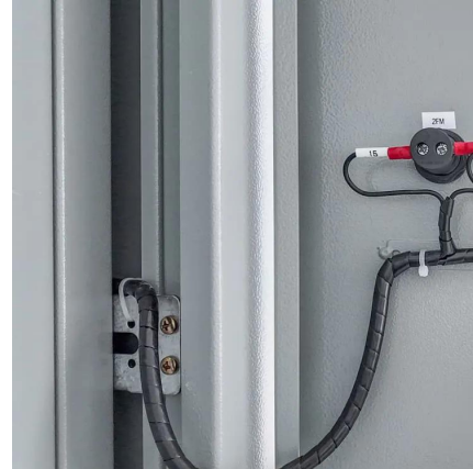
Port Vila communication network cabinet lithium battery ...
