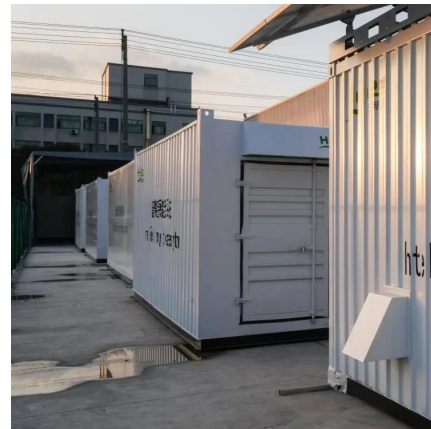
Energy storage container, BESS container
