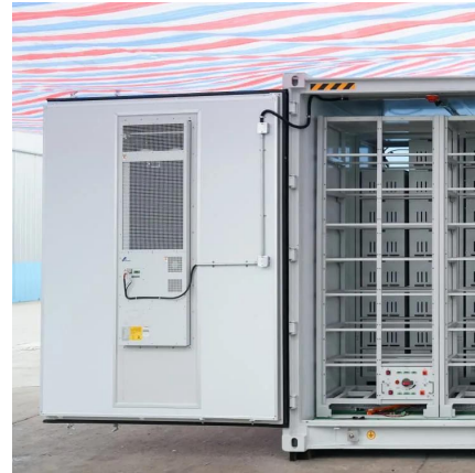
Energy storage container, BESS container
