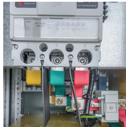
Uninterruptible Power Supply (UPS backup system)
