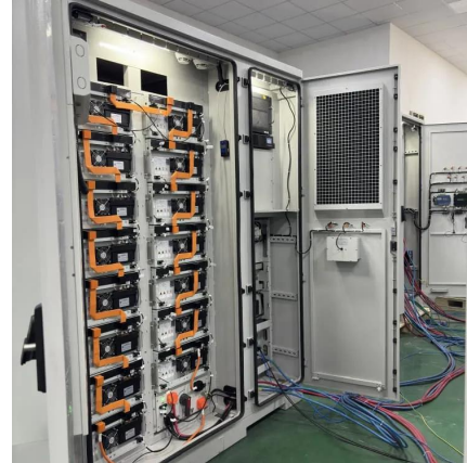
Energy storage power source factory in Gothenburg Sweden
