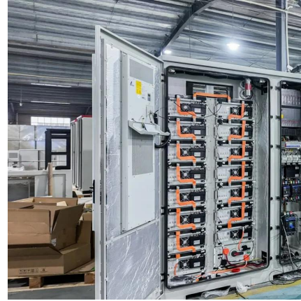
east timor energy storage charging station
