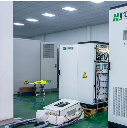
Energy storage container, BESS container
