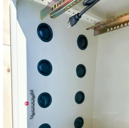
Energy storage container, BESS container
