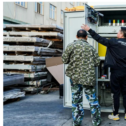
Mobile Energy Storage , Power Edison
